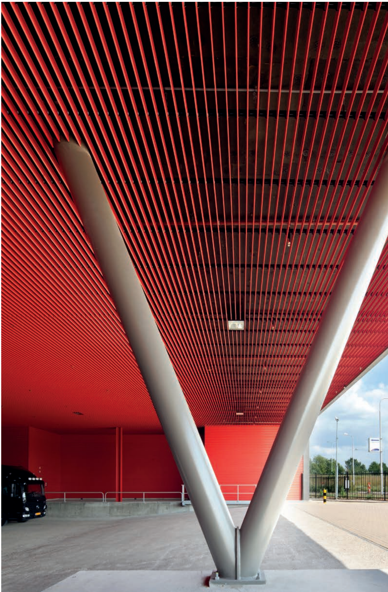
Project: Distributie Centrum, Tilburg, the Netherlands - Product: Baffles V100 - Architect: Jeroen Weijers, Van Oers Weijers Architecten
